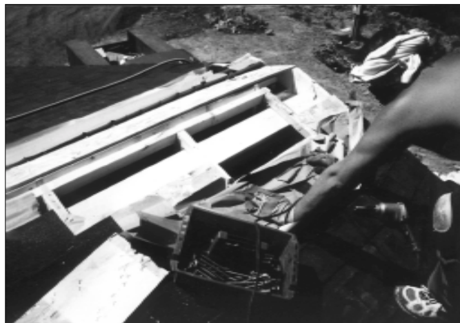
To meet OMDS bolting requirements, factory roofing and additional roof sheathing had to be removed so the ends of the ridgebeams could be bolted.
