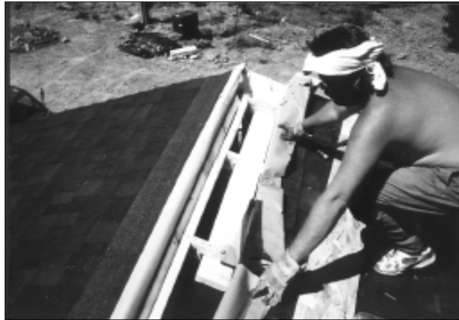
When the last row of sheathing was removed so the ridgebeams could be bolted, a 2x6 outlooker supporting the barge rafter did not allow room for the installer to get his arm or the bolt gun into the roof at the ends of the ridgebeam. See photo below.
