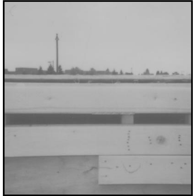
The roof cavity vents through the roof, so the seal is ineffective.
