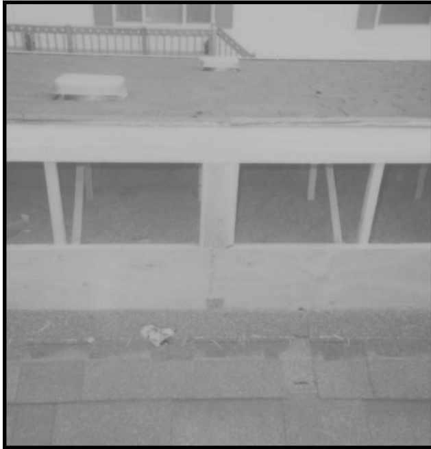
The ridgebeam is not a full beam; the installer placed the seal sill at the upper portion of the assembly.
