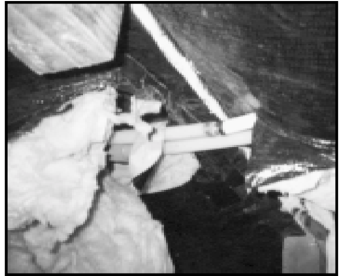
Uninsulated plumbing pipes
