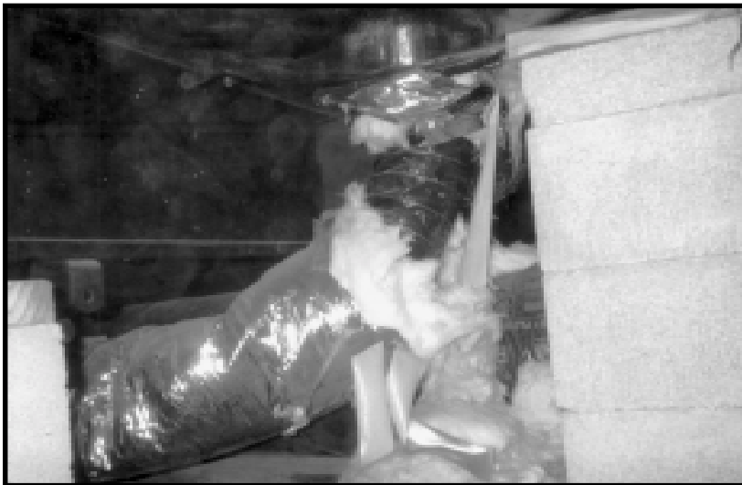
One of the common problems in installations: heat ducts not properly connected
