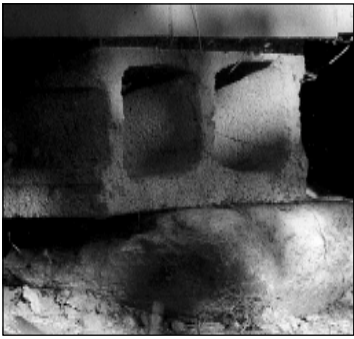
Improper perimeter blocks
